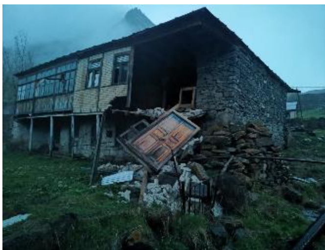
Collapsed house in Tskere
